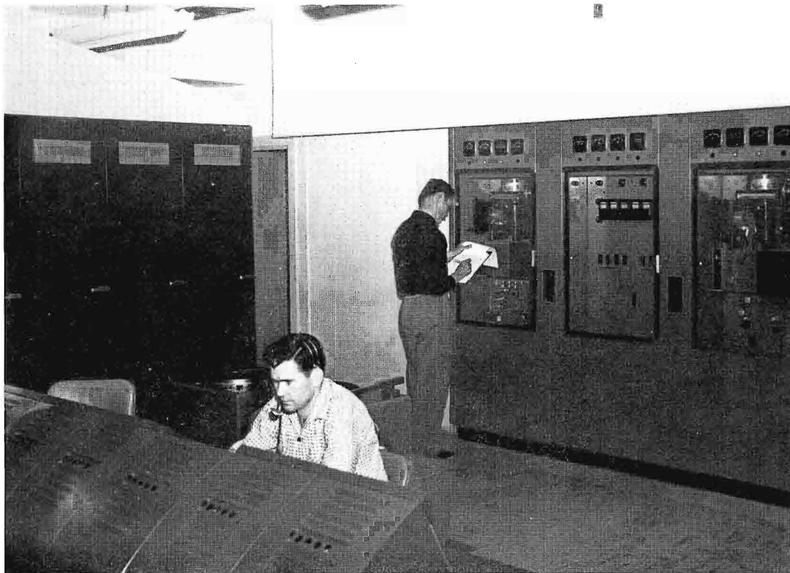
FIG. 11. View of the WJTV transmitter room showing the RCA TTU-1B, 1 KW UHF transmitter and partial view of the console. Note that provision is made for addition of RCA high power amplifier. Harold Townsend is shown at the transmitter and R. K. Somers at the console.
