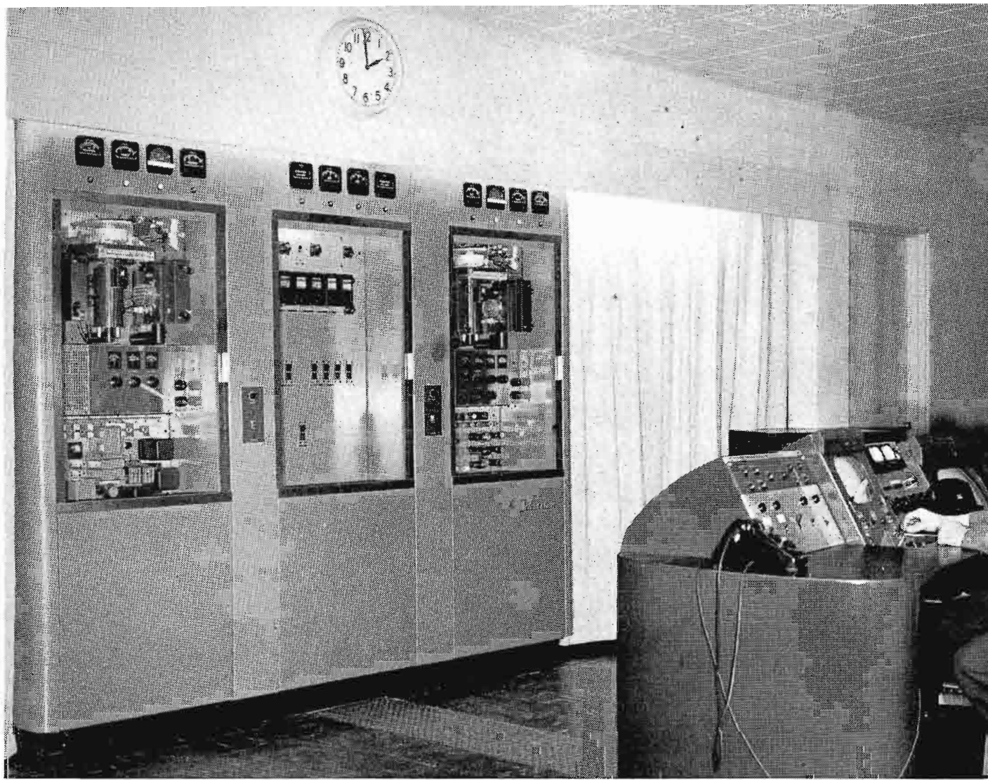
FIG. 2. WHP-TV's Chief Engineer, Dan Leibensperger, is shown at transmitter controls. Transmitter is the RCA TTU-1B.
